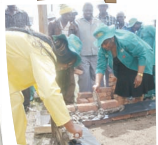
MEC Mashego-Dlamini and HOD Nelisiwe Sithole laying bricks for the construction of a kitchen at God's Will Disable Centre
