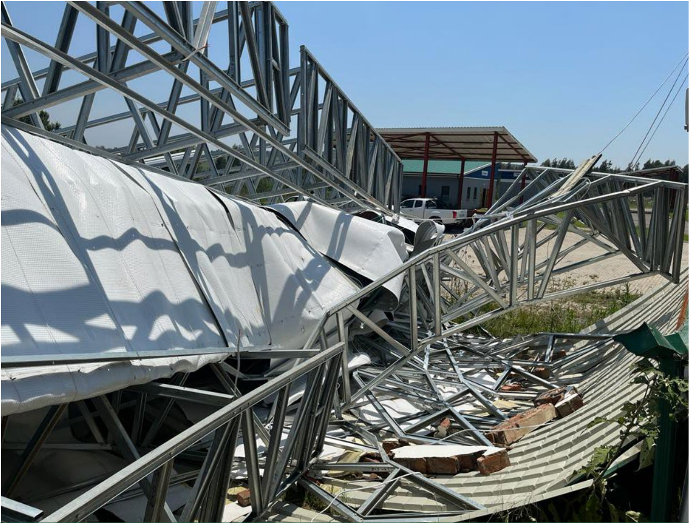
Damage caused on the Mkhondo Agri Hub
